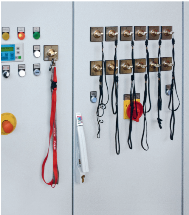
Central control panel with key switch system
